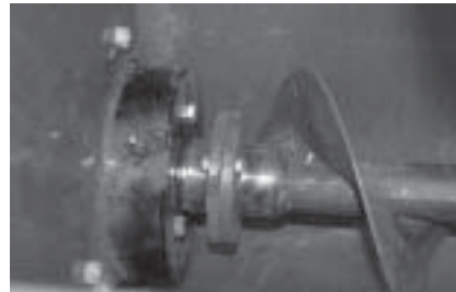
Transfer Auger Front Bearing (under mill cover, 1 zerk on front bearing)
